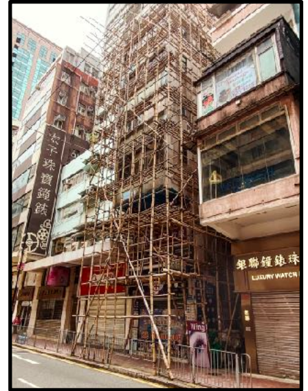
Watching construction in HK is amazing. Workers climbing over scaffolding like this, without tethers or nets. This has always been common practice and why construction moves at breakneck speeds.
